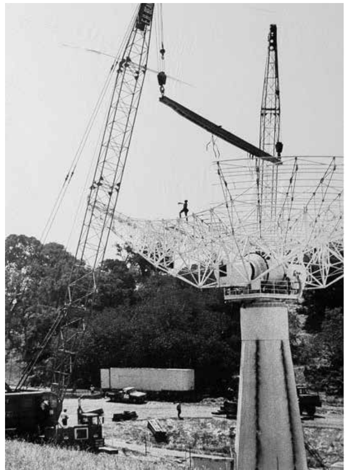
Figure 1. The 27-m ISR antenna at Stanford University, California.
